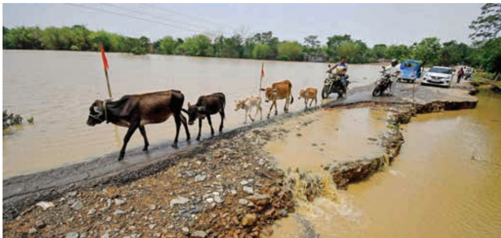
A group of cows walk in a road that got damaged due to heavy rainfall triggered by Cyclone Remal, in Nagaon, Assam on Sunday (ANI)
