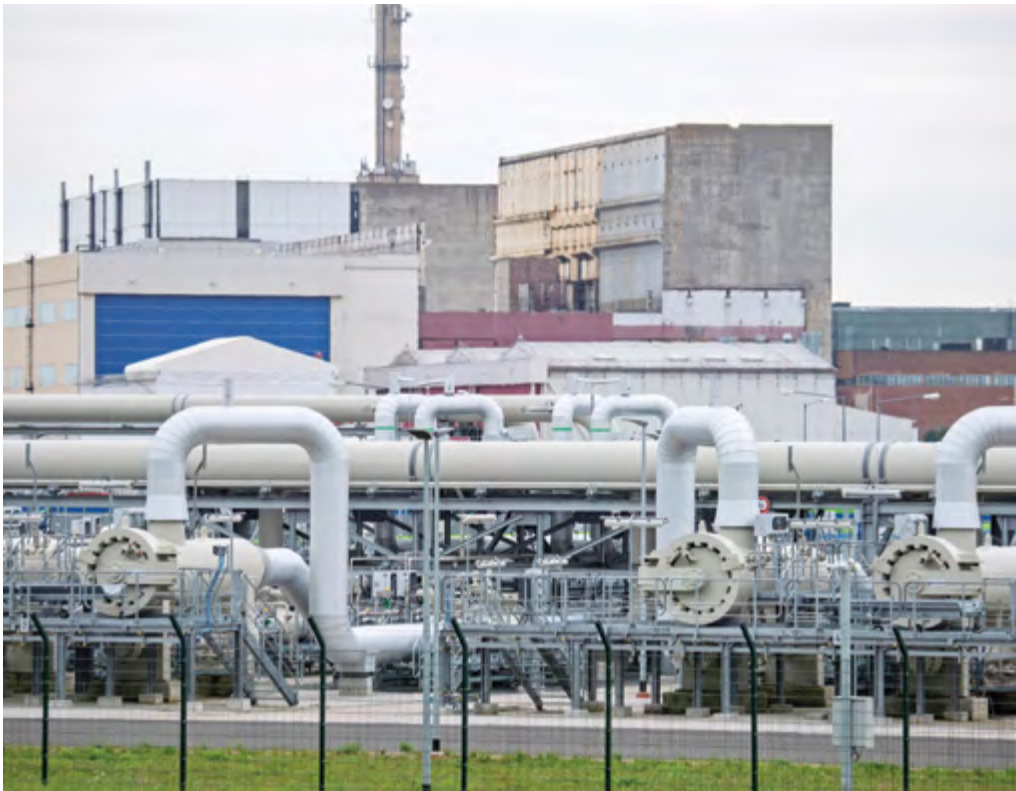
A file photo shows a view of the Gascade Gas Receiving station adjoining the Nord Stream 2 Pipeline Inspection Gauge (PIG) receiving station in Lubmin, northeastern Germany (AFP)
