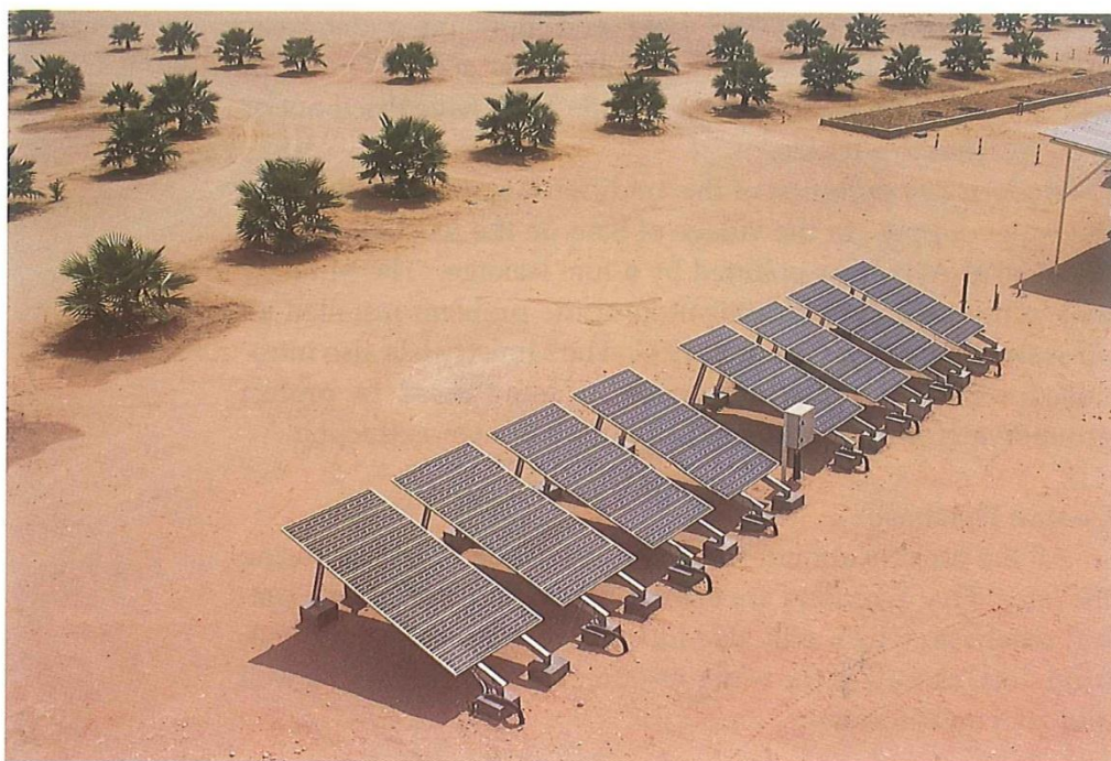
▲ Solar panels are used for raising water from underground aquifers.
