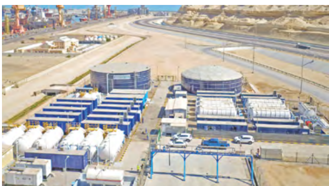
A Marafiq-run water desalination plant in Duqm
