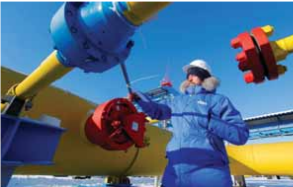
An employee checks a gas valve at the Atamanskaya compressor station, in Siberia. – Reuters
