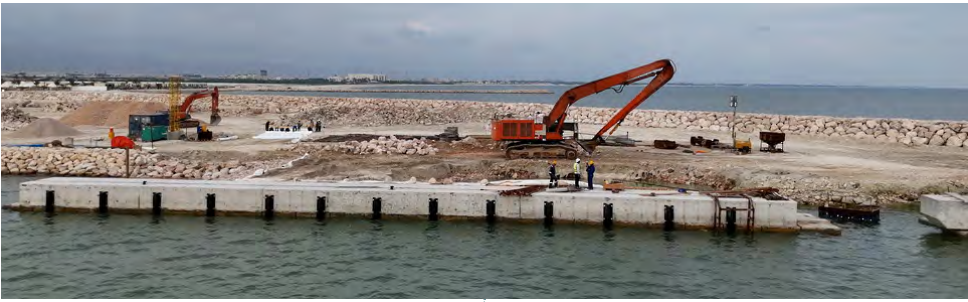
The project forms part of the strategy to enhance the operational efficiency of fishing ports.
