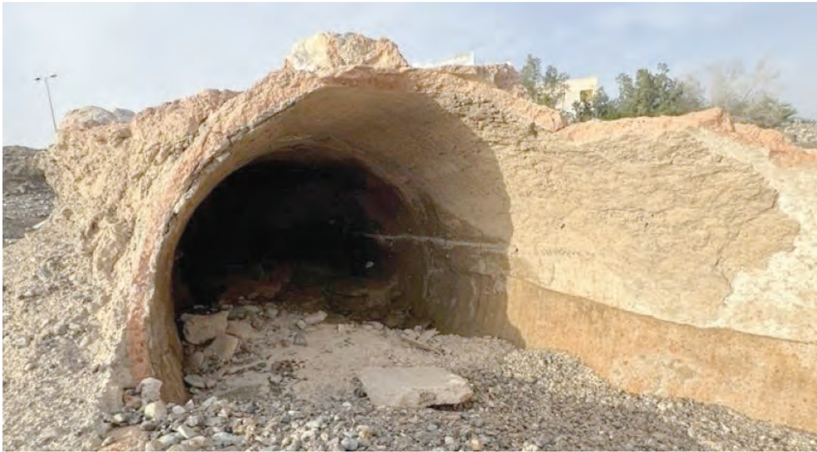
The flash flood triggered by heavy rain washed away some of the debris which caused falaj to appear on the surface
