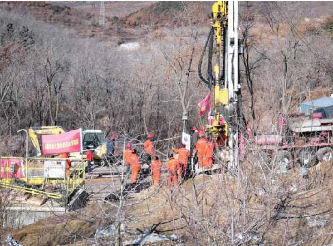
Members of a rescue team work at the site of a gold mine explosion where 22 miners are trapped underground in Qixia, in eastern China's Shandong province. — AFP
