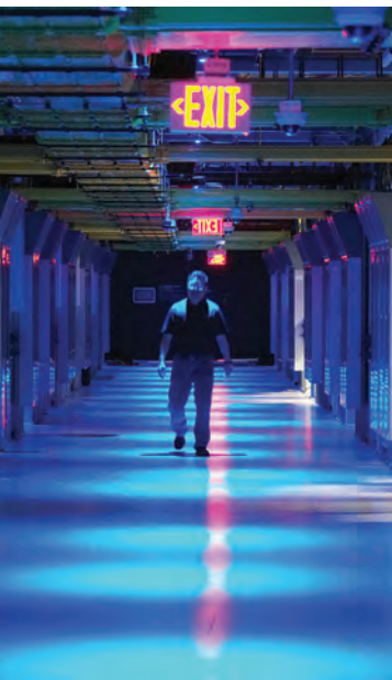
Inside a data centre in San Jose, California.
