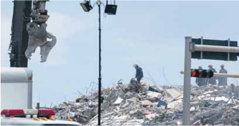
Rescue personnel continue to search the rubble at the site of a collapsed building in Surfside, Florida, north of Miami Beach, on Sunday. — AFP
