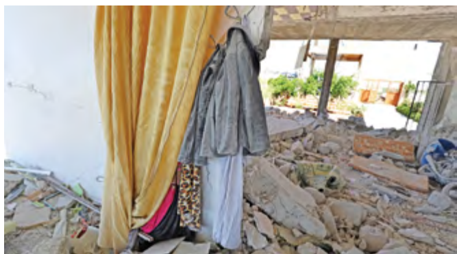
A heavily damaged house in the village of Al-Bara, in the Jabal al Zawiya region of the Idlib province, following the strikes on Monday (AFP)
