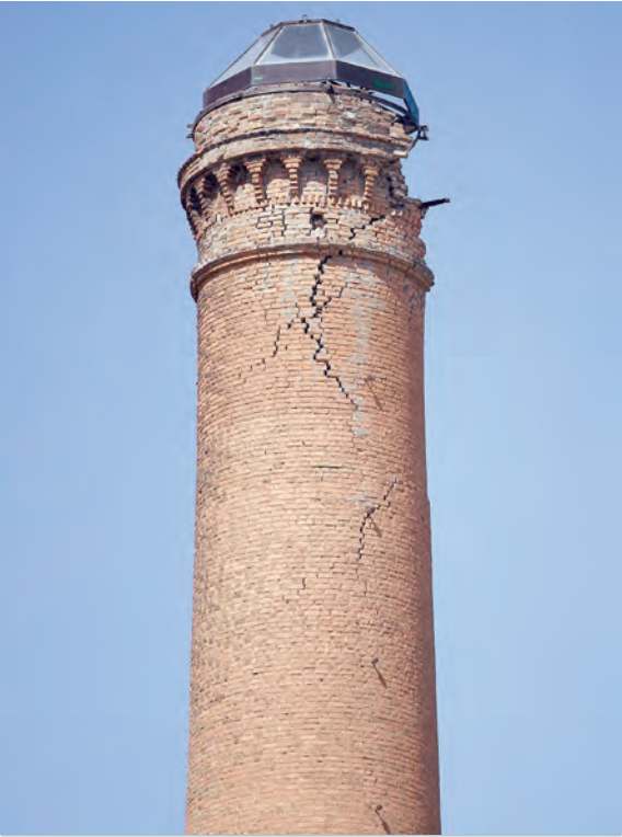
Cracks on a damaged tower in the aftermath of an earthquake that struck southern Spain, in Granada, on Tuesday. — Reuters
