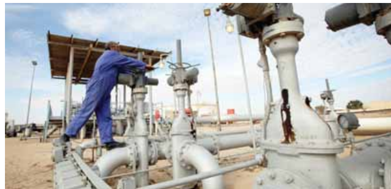
A worker checks pipes and valves at Amaal oil field in eastern Libya. — Reuters
