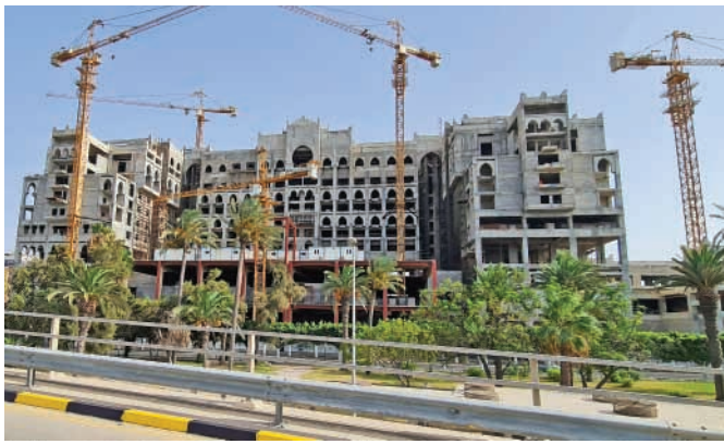
A picture shows an unfinished hotel, after its construction was halted in 2011, in the Libyan capital Tripoli (AFP)
