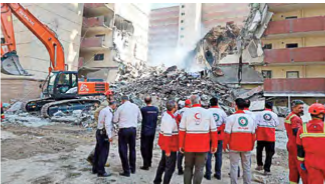
Rescue teams working outside a building that was struck by an Israeli airstrike, in Tehran on Saturday
