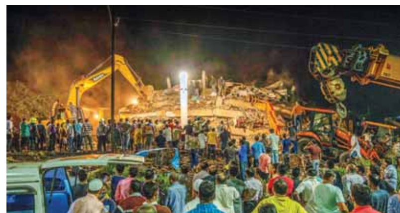
Rescue workers search for people in the rubble of a five-storey apartment building after it collapsed in Mahad. — AFP
