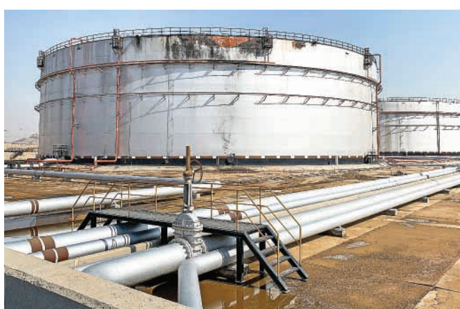
This file photo shows a damaged silo at the Saudi Aramco oil facility in Saudi Arabia's Red Sea city of Jeddah (AFP)
