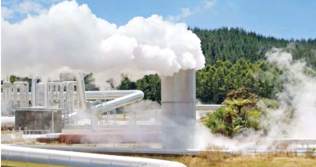
Germany has announced plan to increase production of geothermal energy tenfold by 2030 to 10 terawatt hours
