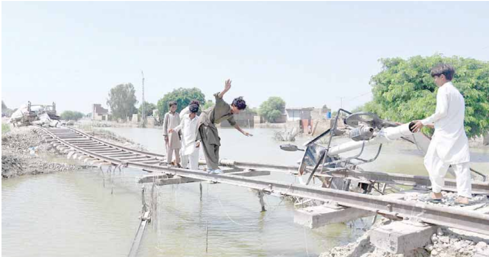
Flood affected residents cross a railway track damaged by flood waters in Fazilpur area following heavy monsoon rains in Rajanpur district, Punjab province. — AFP
