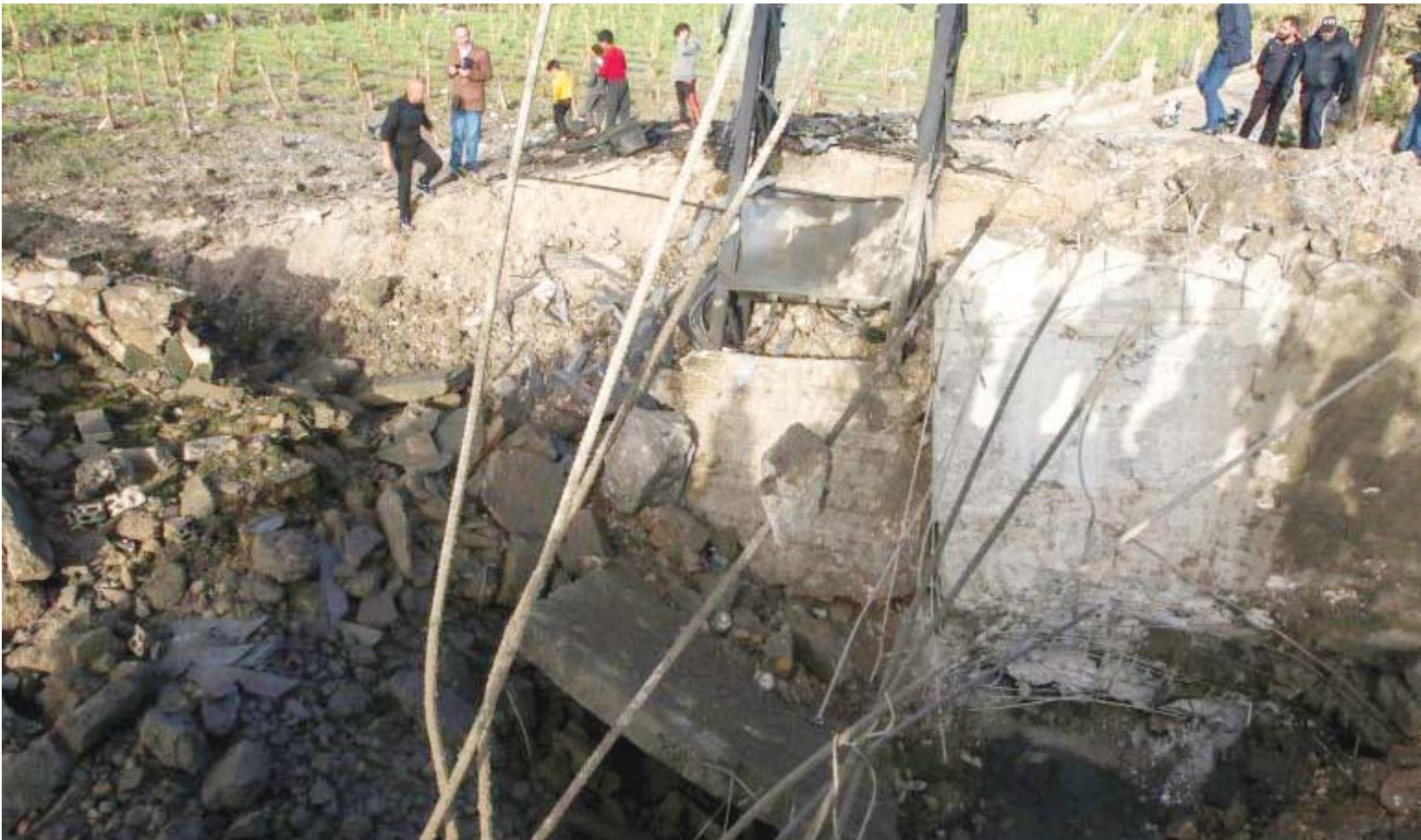
People check a damaged bridge following Israeli air strikes in Al Qulaylah, on the outskirts of Tyre, Lebanon. – AFP
