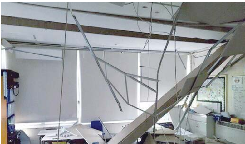
The Department for Education began reviewing the risks posed by RAAC in 2018 when the roof at a primary school in Gravesend, Kent, collapsed
