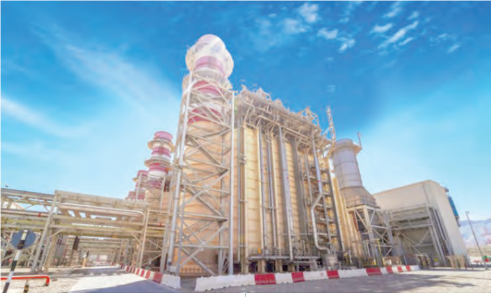
Both gas-powered plants at Misfah and Duqm will be designed to be hydrogen-ready for the first time in Oman's power sector (Picture for illustration only).
