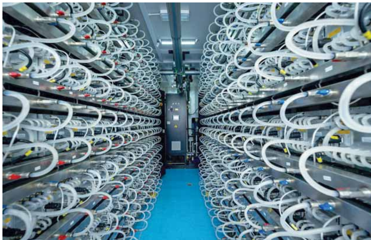
Exahertz's blockchain data centre in Salalah based on BITMAIN's hydro-cooling mining technology.
