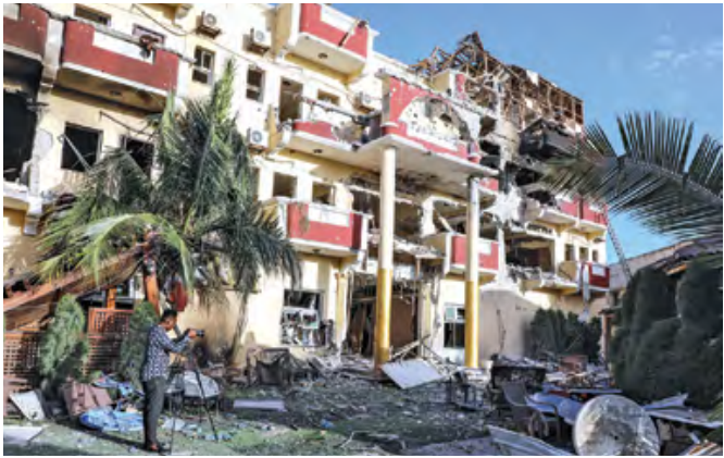
The damaged structure of the Hayat Hotel in Mogadishu (AFP)
