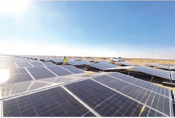
Solar panels now power parts of the main infrastructure works at the Special Economic Zone at Al Dhahirah, supporting road and drainage construction.
