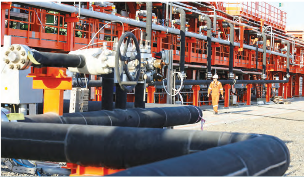
A worker walks past infrastructure on D Island, the main processing hub, at the Kashagan offshore oil field in the Caspian Sea in western Kazakhstan
