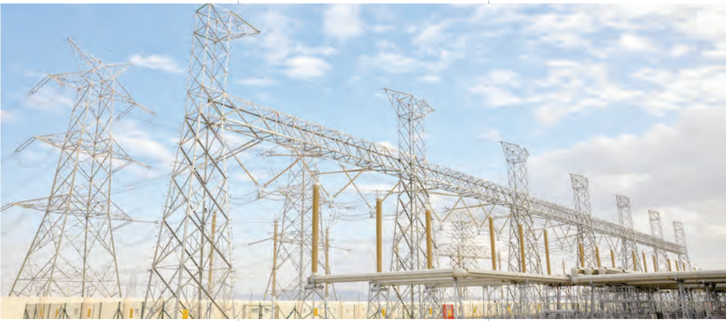
New grid stations will help integrated wind farms and a gas-fired power project into the national grid.
