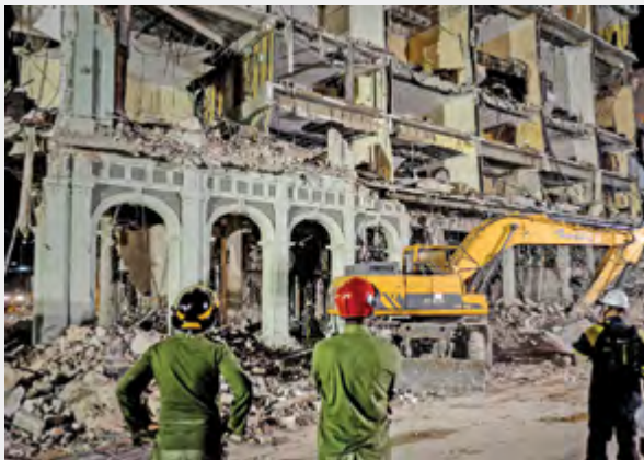
Firefighters and rescue workers remove debris from the ruins of the Saratoga Hotel, in Havana, on Friday (AFP)
