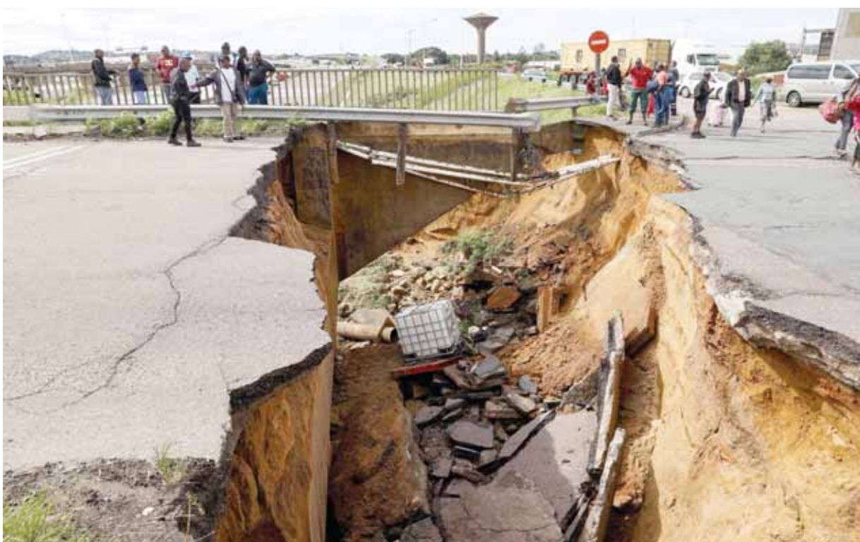
A view of a crack in the road following heavy rains and winds in Durban. — AFP
