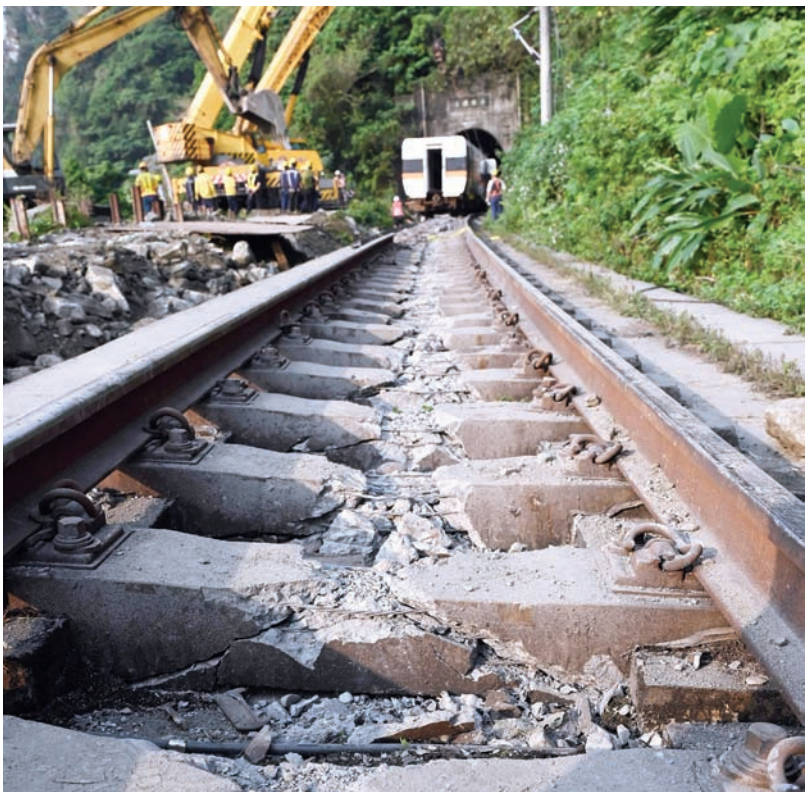
Damaged railroad tracks are seen at the location where a packed train collided with a vehicle on the tracks and then derailed inside a tunnel in the mountains of Hualien, eastern Taiwan. — AFP
