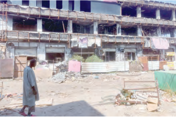
A man walks past a damaged building in Wad Madani, which was retaken by the Sudanese army a month earlier, in Sudan's Al Jazira state. — AFP
