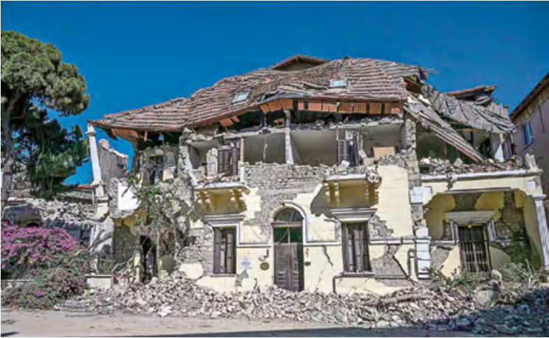
A damaged historical hotel five months after the 7.8-magnitude jolt and its aftershocks wiped out swathes of Turkey's mountainous southeast
