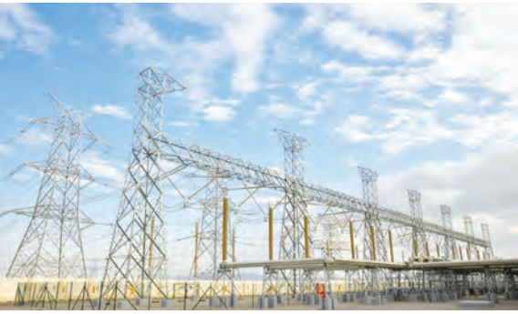
NEDC's RO 154 million investment is designed to strengthen Oman's power grid for the future.
