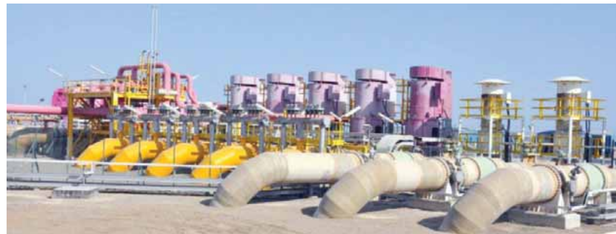
View of Majis' water services infrastructure at Sohar Port
