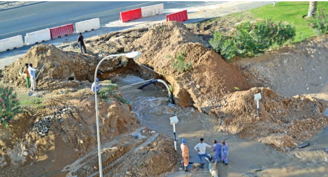
A water pipeline burst near Amerat roundabout on Monday creating a pool of water. The waterflow caused a minor traffic congestion on the adjacent road (Muscat Daily)
