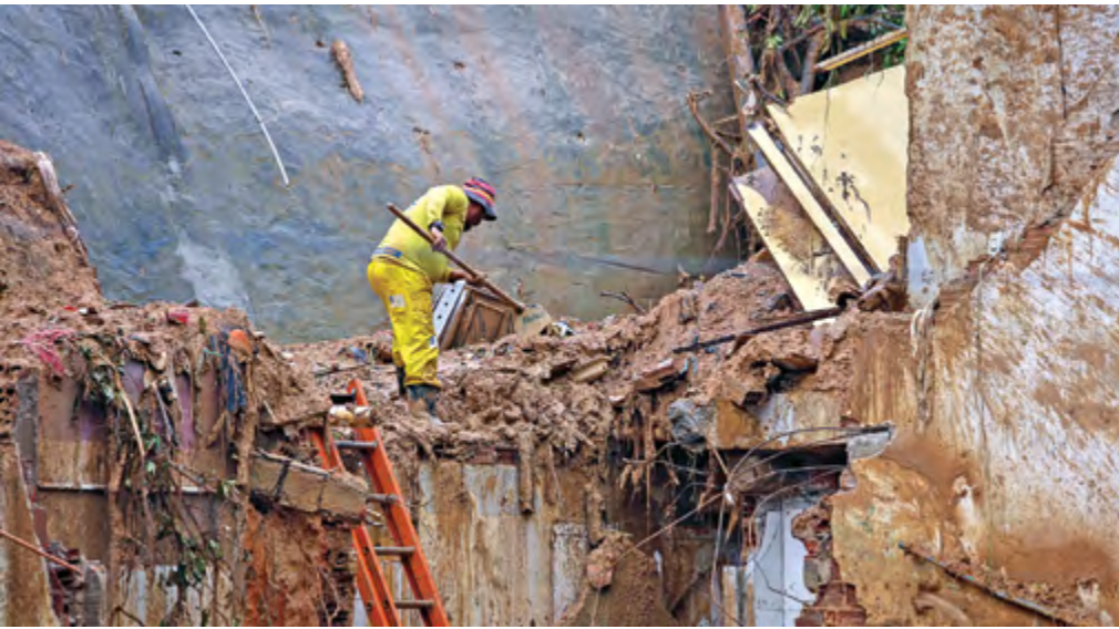
A man removes debris on a landslide area at the community Jardim Monte Verde, Ibura neighbourhood, in Recife, Pernambuco State, Brazil, on Sunday (AFP)
