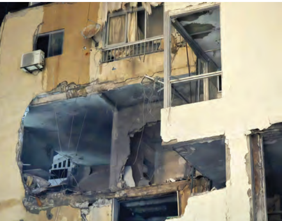
This picture shows the damage following an Israeli strike in the southern Lebanese city of Tyre. — AFP
