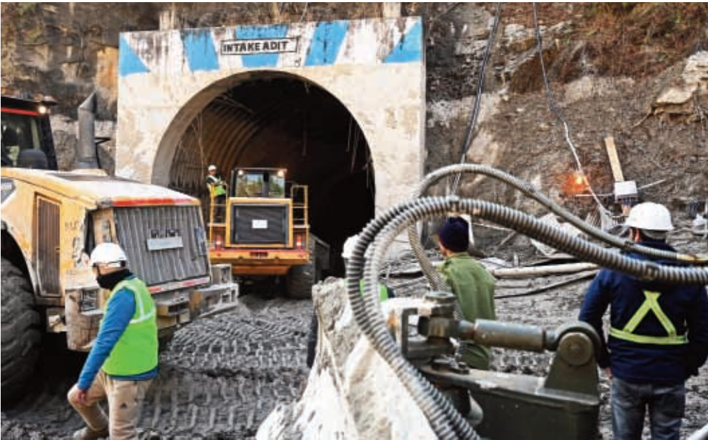
Rescue teams outside the entrance of a tunnel in Chamoli district on Wednesday where dozens are still feared to be trapped following a flash flood thought to have been caused when a glacier broke off three days ago (AFP)
