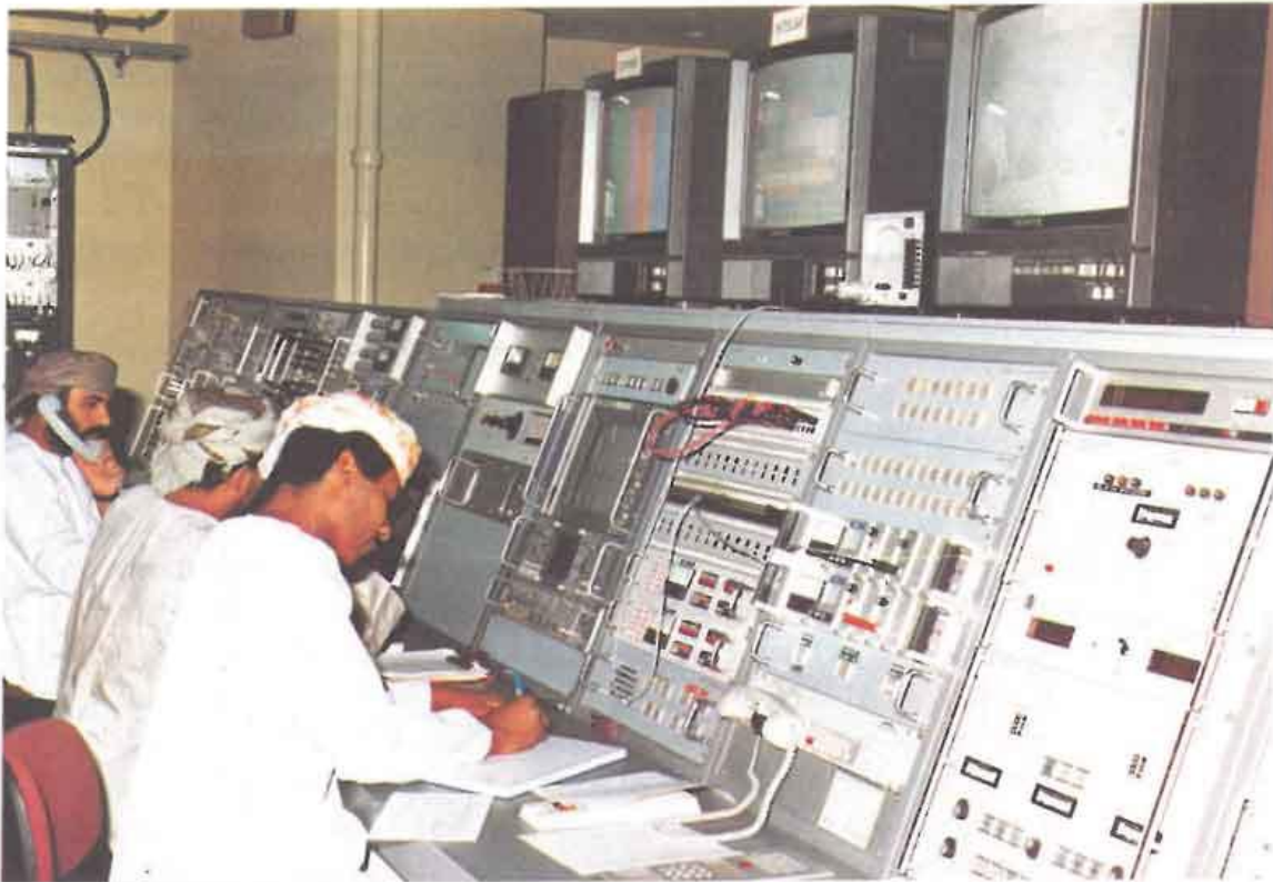
The central console at Al Amerat which controls Oman's satellite telecommunications complex (Photo: Ministry of Posts, Telegraphs and Telephones)
