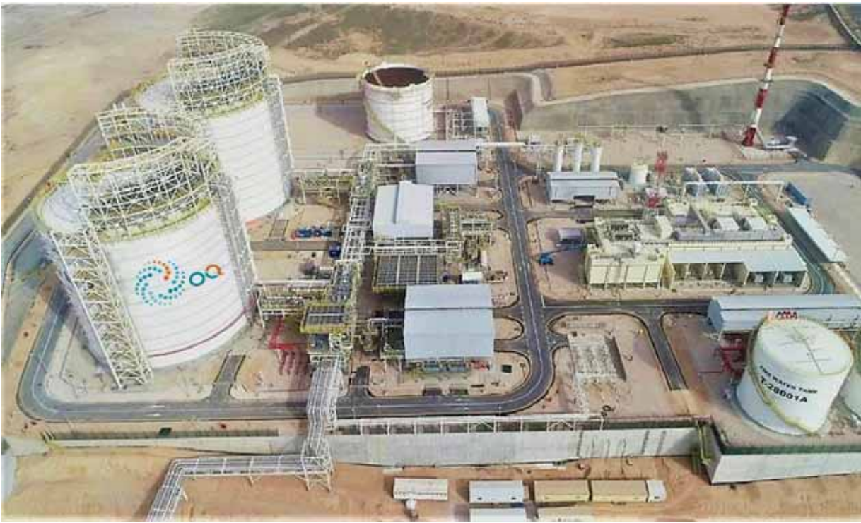
The centrepiece of the project is an extraction and fractionation plant designed to process up to 8.8 million standard cubic metres/day of natural gas
