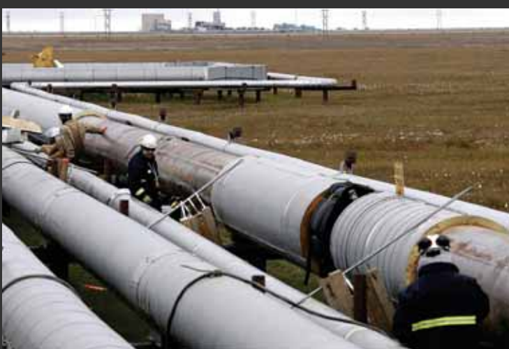
BP workers are seen at an oil transit pipeline at the Prudhoe Bay oilfield in Alaska. — Reuters
