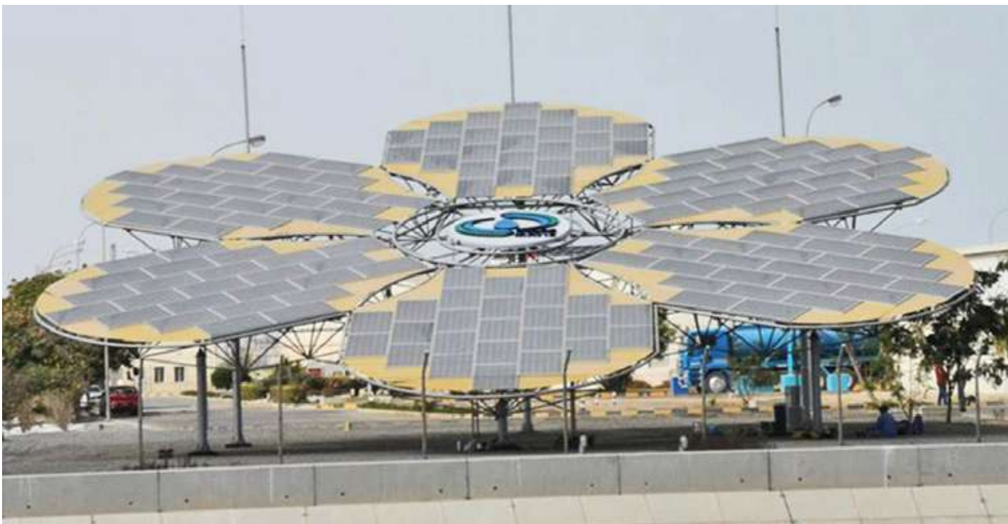
150 SOLAR PANELS: In terms of design, the project consists of 150 solar panels within 300 square metres. - ONA
