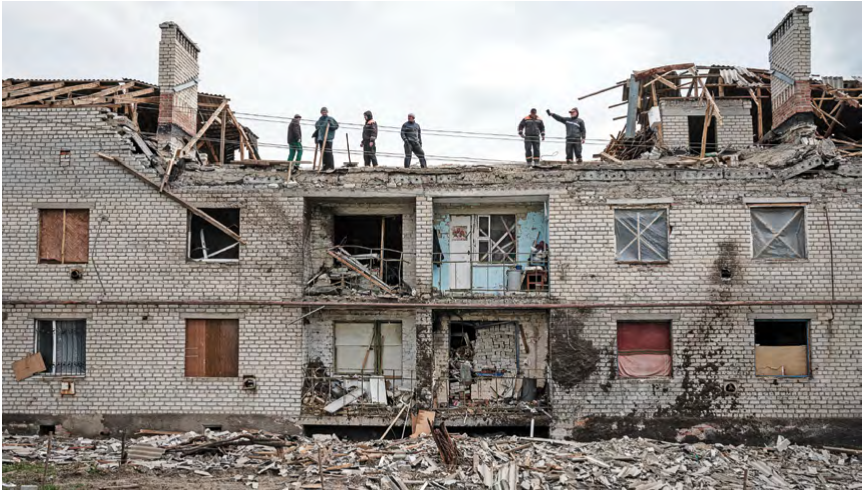
Workers clean rubbles atop a building destroyed by shelling a month ago in Cherkaske, eastern Ukraine on Wednesday (AFP)
