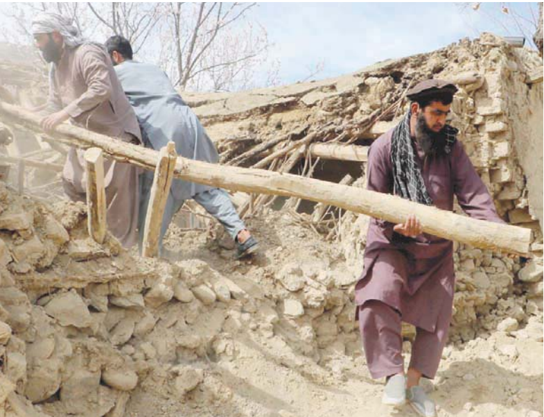
Residents clear debris from a damaged a house at Sooch village in Jurm district of Badakhshan Province in Afghanistan. — AFP
