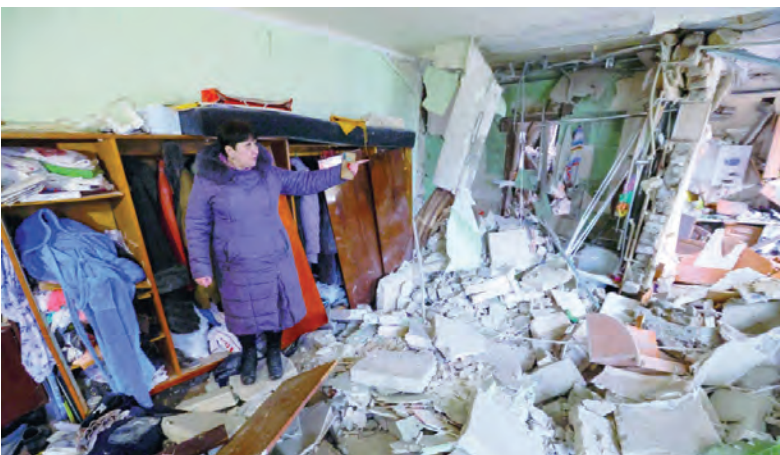
Local resident Viktoria stands amid debris of her apartment in a building heavily damaged in recent shelling in the course of Russia-Ukraine conflict in Horlivka (Gorlovka) in the Donetsk region, Russian-controlled Ukraine, on Wednesday.
