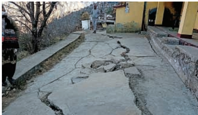
A view of damaged pavement due to landslides, in Joshimath (ANI)
