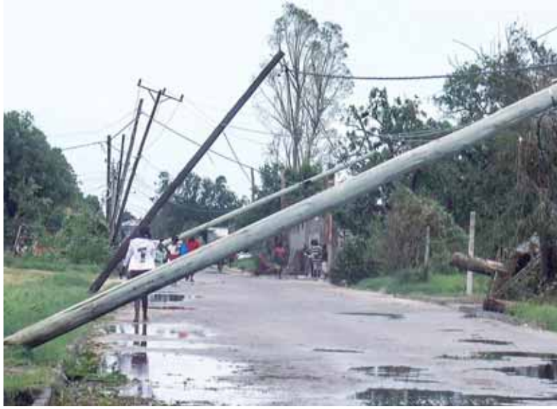
An image taken from an TV video shows fallen utility poles in a street of the port city of Beira after Tropical Cyclone Eloise hit Mozambique. — AFP
