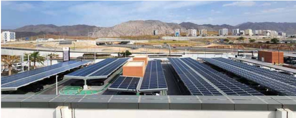
Solar PV installations on the rooftops and carports of Mall of Oman.
