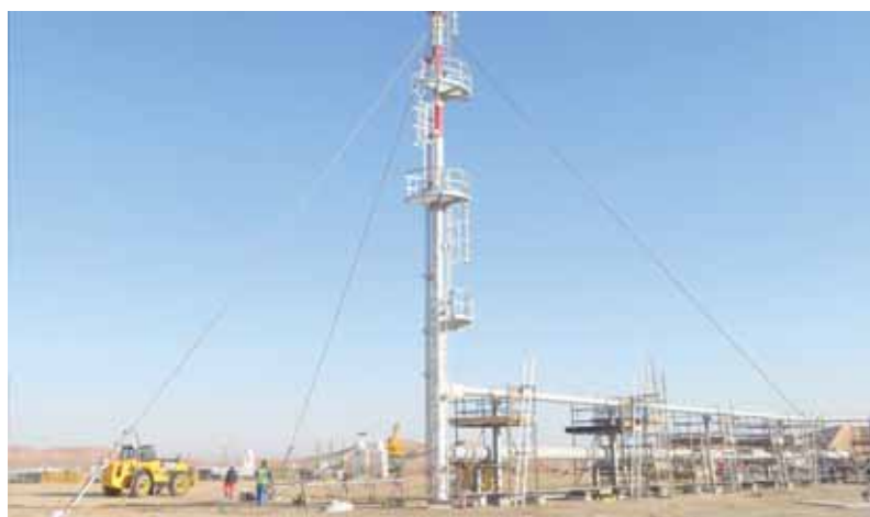
Mitigation of routine flare, GHG emissions and methane leaks is a key priority.
