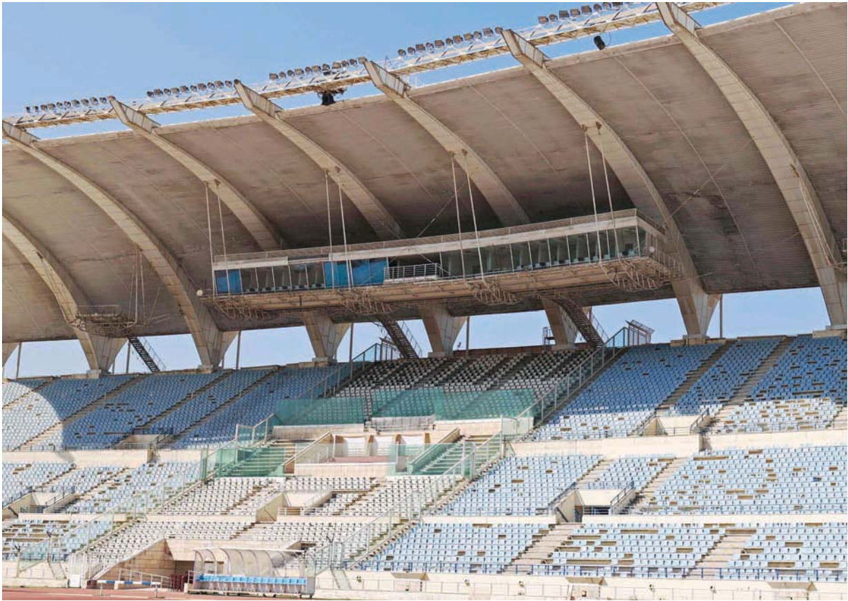
A partial view shows the deterioration of Camille Chamoun Sports City Stadium in Beirut on Friday. — AFP
